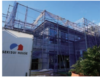
New Sekisui House construction that includes HED-Net system (Photo: Matsudo, Chiba, November 2020)
