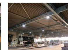
Switching to LED lighting (steel inspection area)
