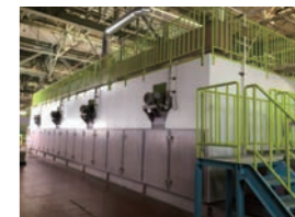
Insulation on the exterior of a drying furnace
