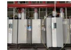
Latest highly-efficient boiler
